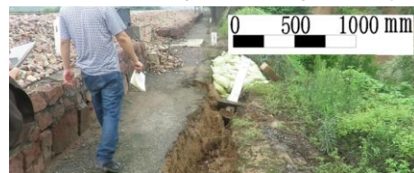
图3 铁路水害沿线某路堤滑坡后缘拉张裂缝 Fig.3 Tension crack on trailing edge of an embankment landslide along water damaged railway
